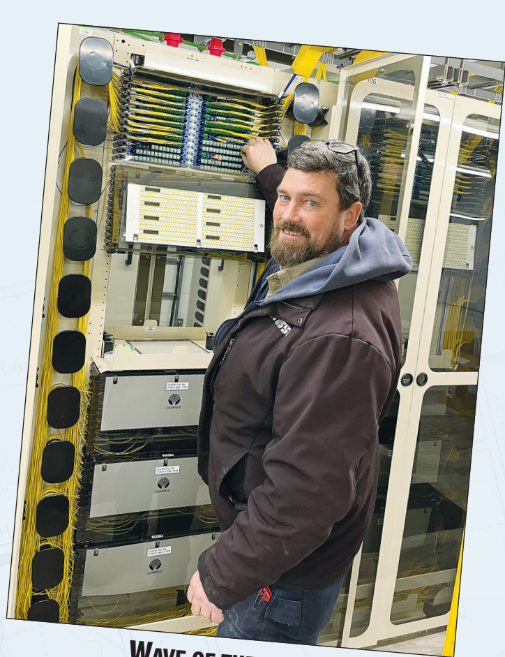
WAVE OF THE FUTURE NEW HAMPTON MUNICIPAL UTILITIES GENERAL MANAGER BRIAN QUIRK AND HIS STAFF HAVE BROUGHT STATE-OF-THE-ART TELECOMMUNICATIONS TO NEW HAMPTON PAGE C3
